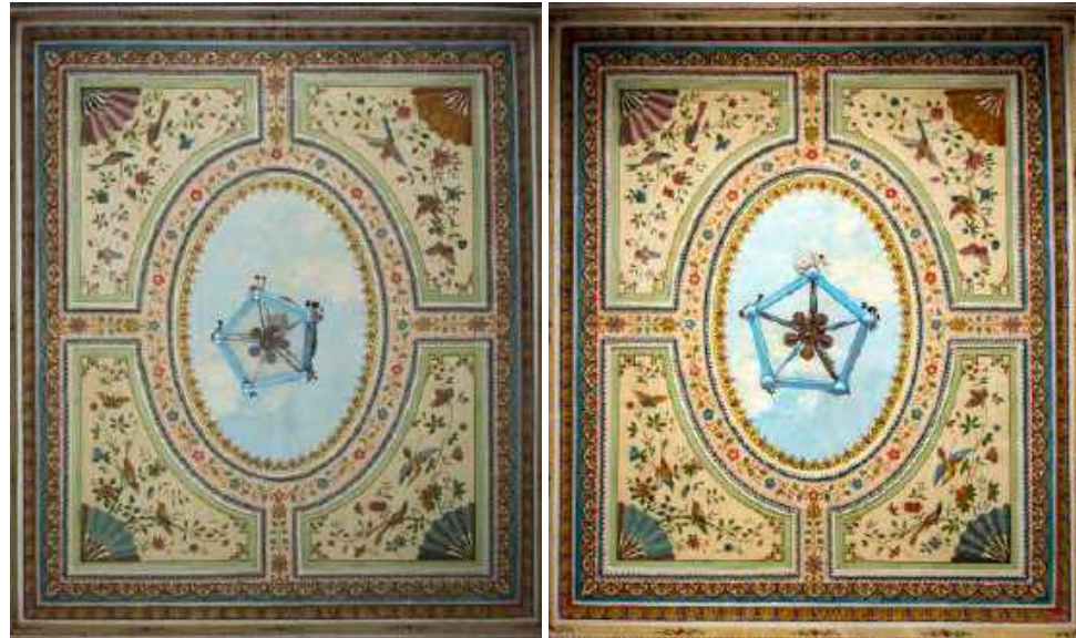
View of the ceiling painting depicting the sky with Chinese fan decoration in each corner, foliage, and birds, before and after restoration.
